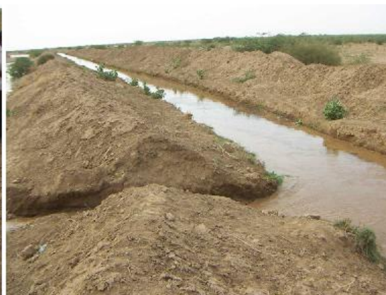
Fig. 7 Cutout of the canal bank to let water flow to farm fields
