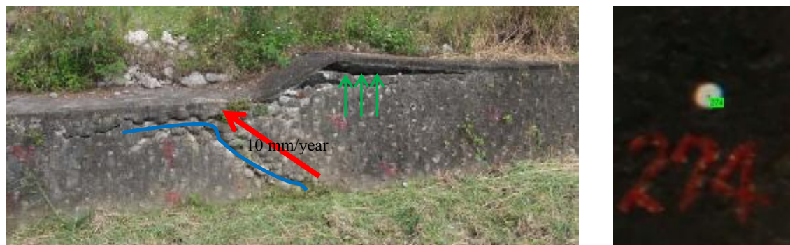
Figure 1 (a) Rupture surface and relative displace direction; (b) The permanent targets on the wall
