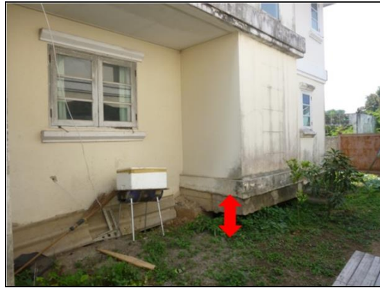
Figure 1. Slip-up phenomena observed in Bangkok. The red arrow shows the slip-up, a gap between the building base and ground.
