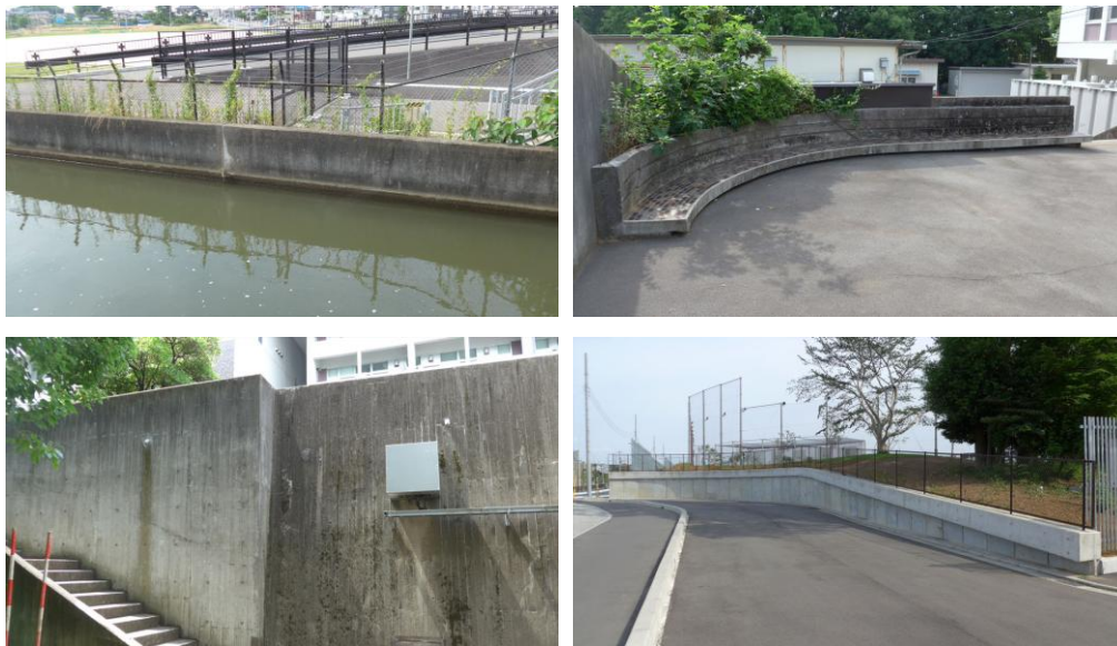
Figure 8. Measured objects (upper left: revetment; upper right: concrete bench; lower left: retaining wall (1); lower right: retaining wall (2))
