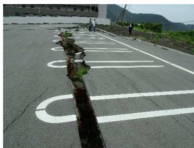
(b) Crack in a parking area
