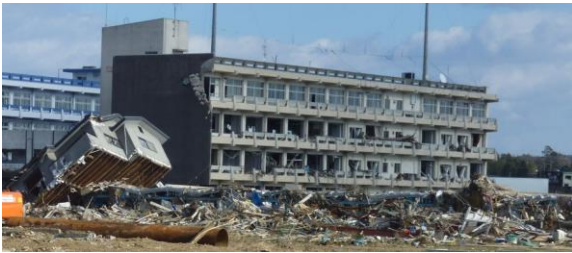
Figure 5. Outlook of Kesennuma-Kouyou High School after the tsunami.
