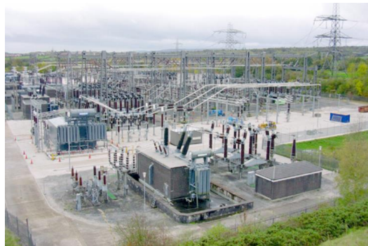
Figure 1. Photograph of a large-scale substation, highlighting its complexity and significance in modern electrical systems (Captured from a figure in Energy Education, 2024).
